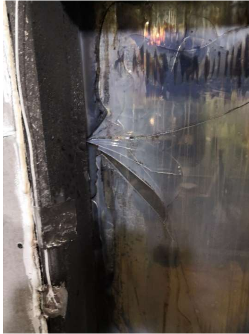
Figure 46 - TGU-T4 fractured glass
