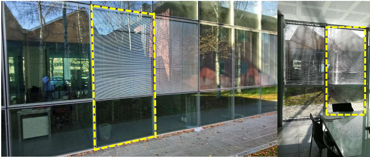
Figure 50: Focchi Headquarters meeting room monitored
